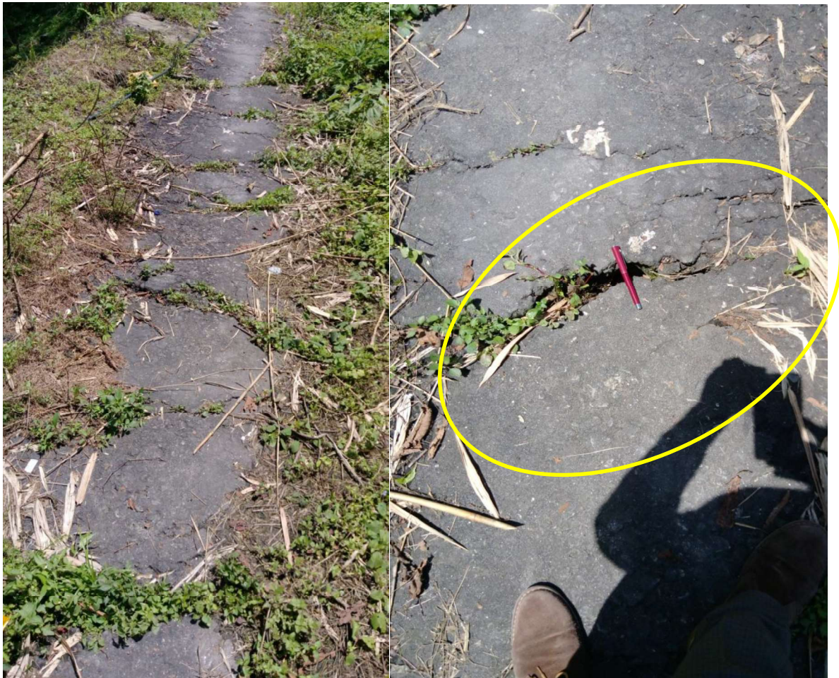
Fig 9: Showing cracks in the road in the slide zone below SNT complex
